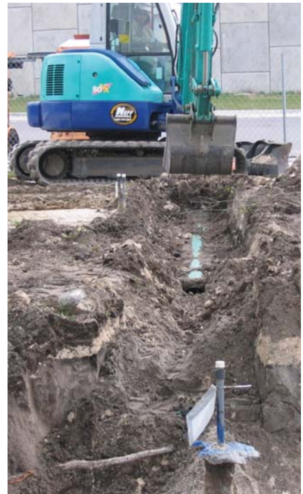
Figure 3 shows a floor drain system that was unearthed during excavation of 94 tons of soil. This was considered the source of the contamination.
